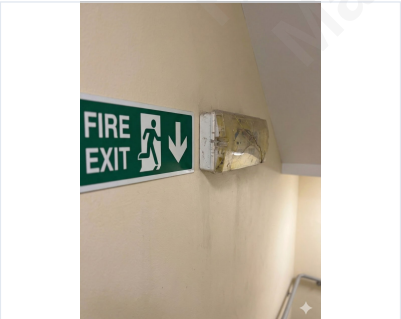
Photo evidence for Emergency Lighting
